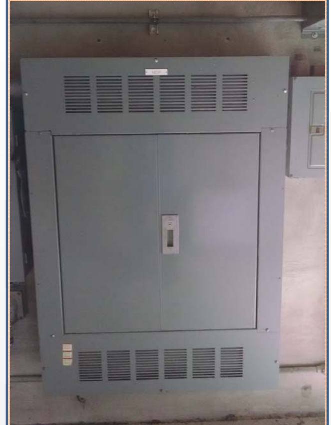
Existing Electrical Power Controls Smith Engineering Contract
