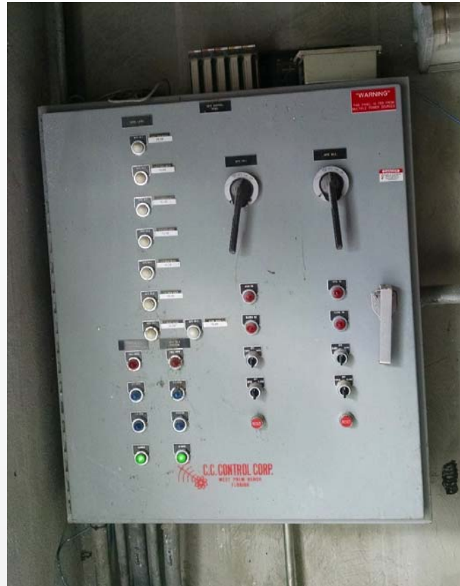
Existing Gate Control Panel
