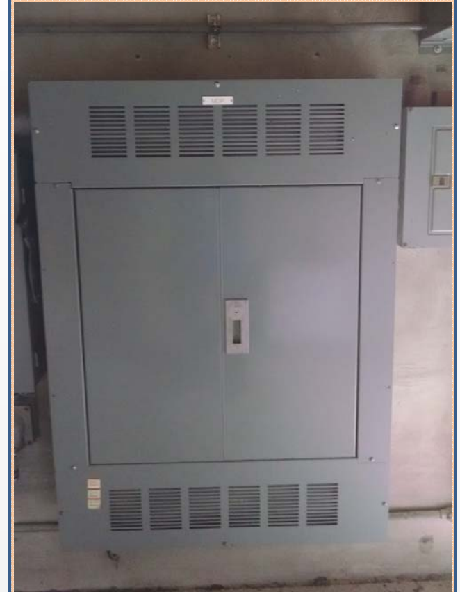
Existing Electrical Power Controls Smith Engineering Contract
