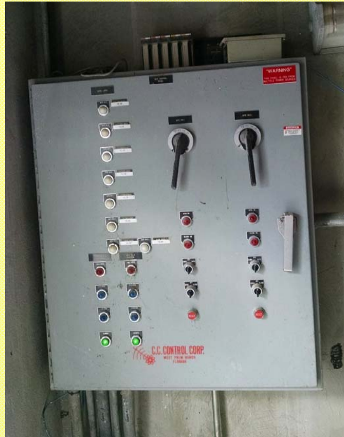
Existing Gate Control Panel
