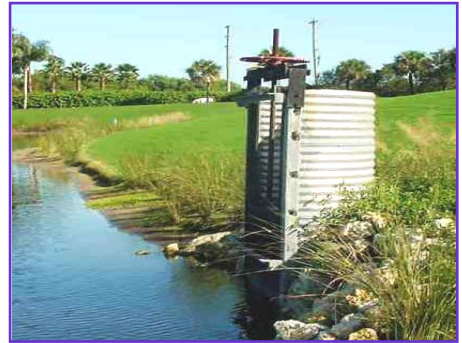
Operable Discharge Control Structure
