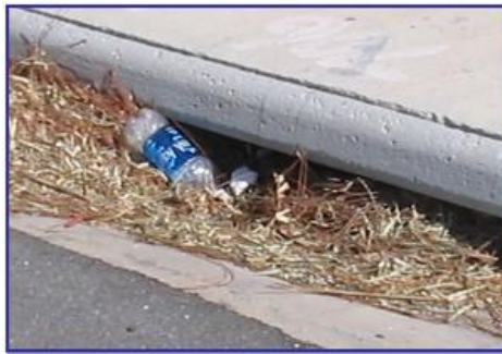
Blockage of vegetation and trash
