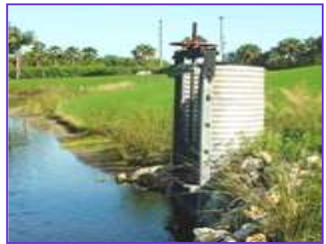
Operable Discharge Control Structure
