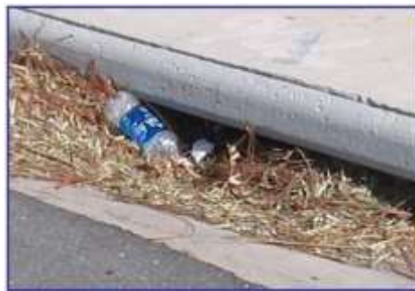
Blockage of vegetation and trash
